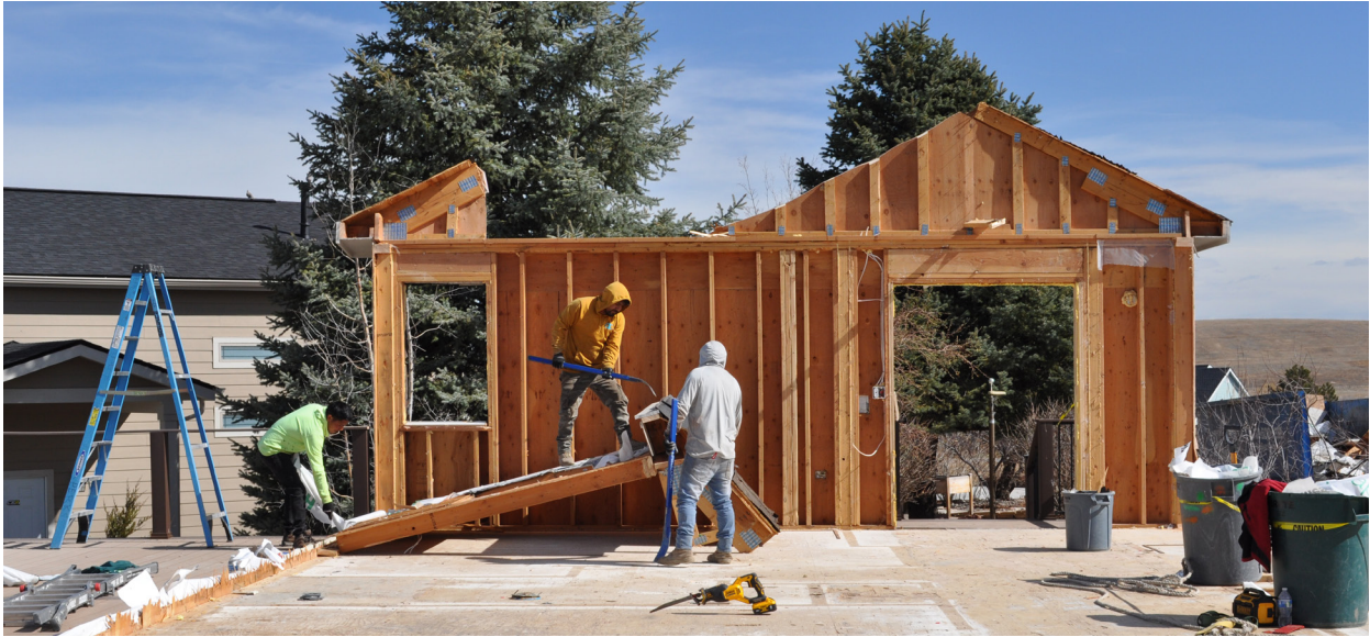
Deconstruction project by Perks Deconstruction, a nationally recognized leader in deconstruction based in Commerce City, Colorado
